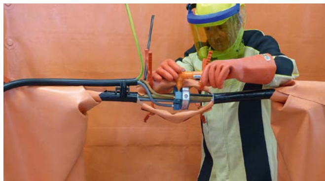
Covering live parts.
