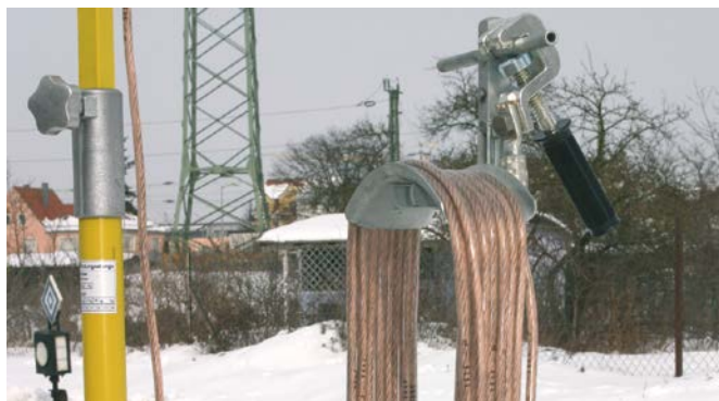
Earthing spike with coiled earthing cable.
