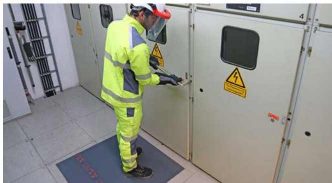
Switch room with insulating mat fitted.
