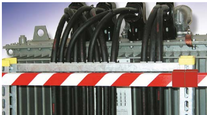
Barrier in a transformer station.
