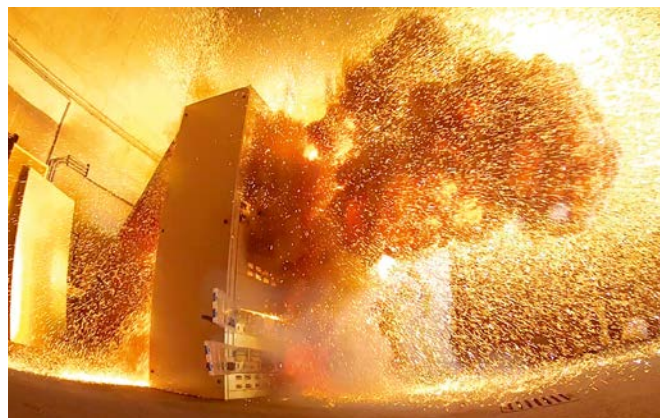
Arc fault accidents can be avoided.
